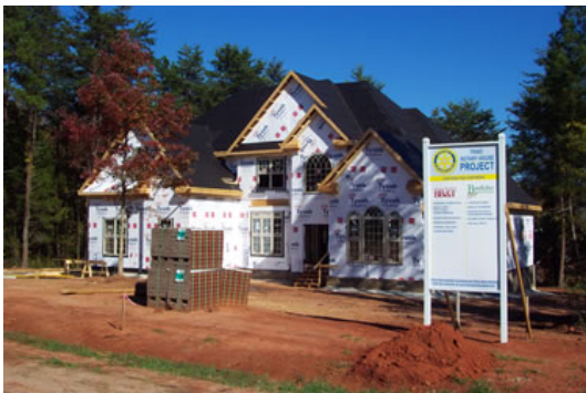
This photo, taken on October 20th, shows the newly-added roof and windows. Shingles are next!
